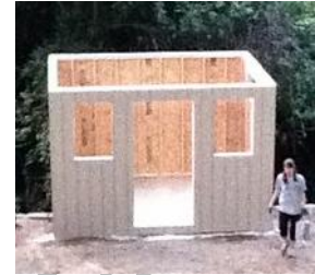
The above picture is of our walls, framed and sided. Emily is already at it working on the garden, and pointing out my mistakes! Quality Assurance is a good thing!
