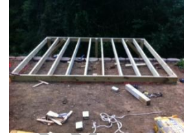
The above picture is our floor framing prior to installation of cross-bracing. There are about 8 piers cemented ~4' into the ground.
