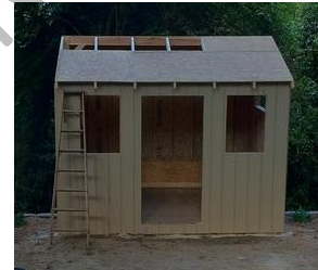
The above picture is after installing the ridge board, the rafters, and beginning the sheathing of the roof.
